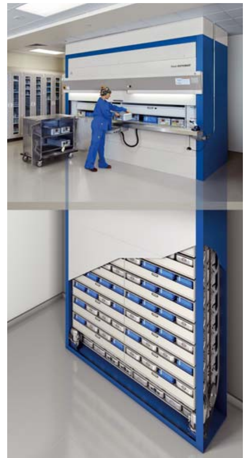
One Rotomat® installed near the operating rooms is in a 20 ft / 6 m deep shaft. The system's total height is 26 ft / 8 m
